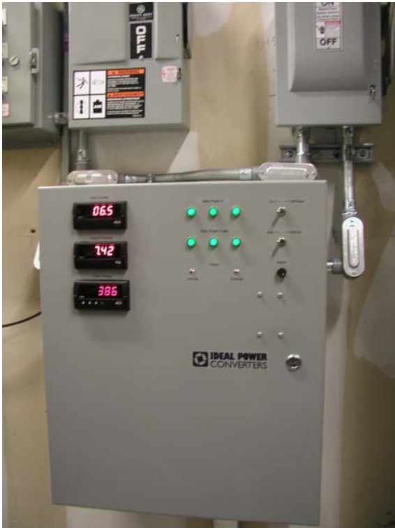
Figure 1. IPC 15hp VFD System in Pilot Testing
